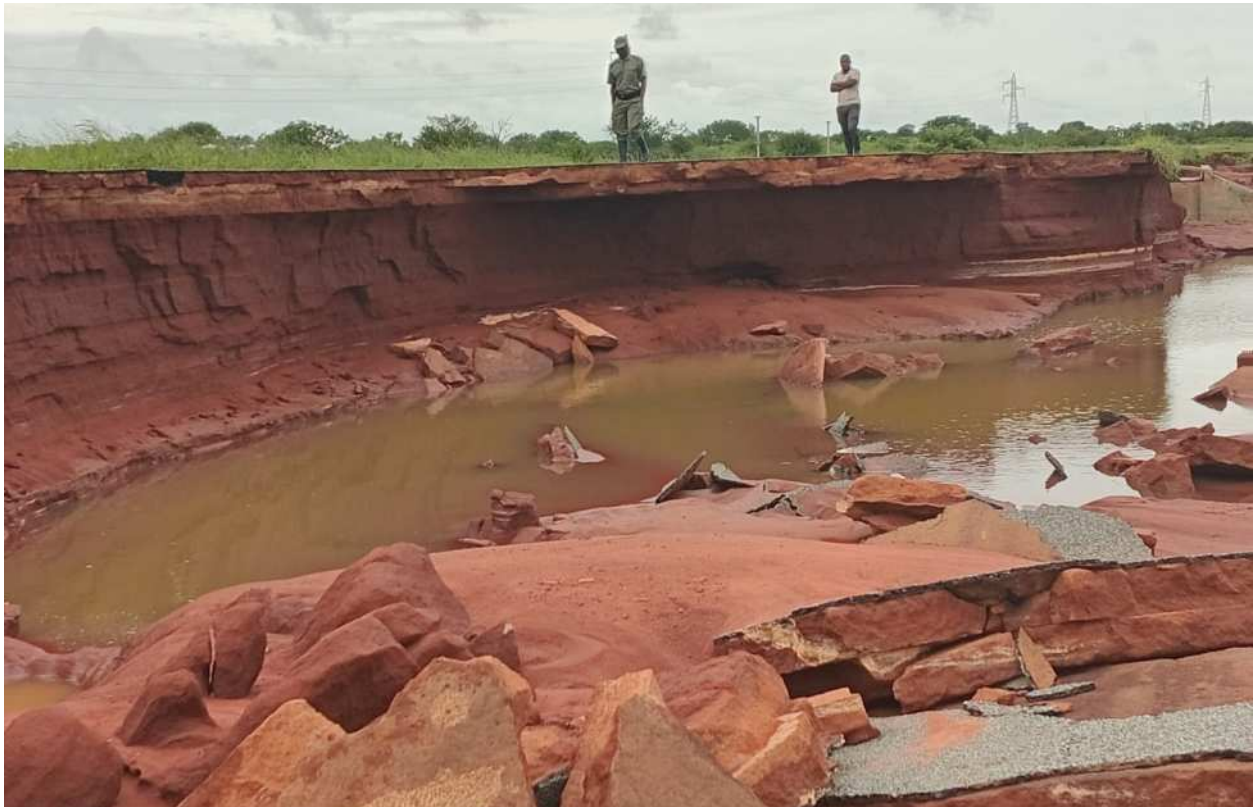
Roads, including the national highway, were severely damaged by the floods.
